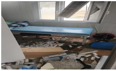
Image 8: A destroyed treatment room
