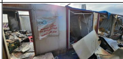
Image 3: The destroyed entrance area
